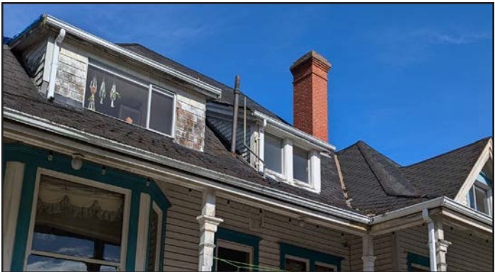
Figs. 37 and 38: (Top) Northwest corner roof, 2024, showing deterioration and excessive moss growth. (Bottom) South facing roof, 2023, showing the deteriorating roof, in particular the missing flashing. (Sources: Cummer)
