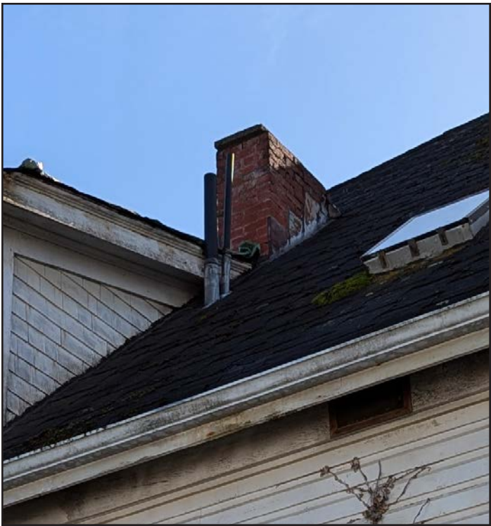
Fig. 39: Northeast corner of Annandale, 2024, showing the chimney remnant missing its top half. (Source: Cummer)
