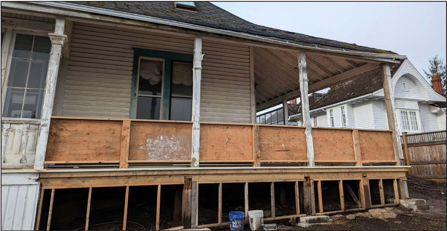
Fig. 40: Northeast corner view of Annandale, 2023, showing the rotten beams and the temporarily stabilised portion of the verandah. Note the deteriorating roof and drainage system, with the gutter peeling away from the building. (Source: Cumber)
