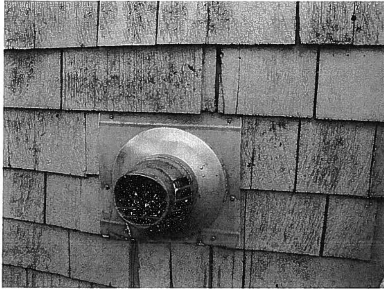
Detail of shingle siding. Note shingles that are cracked and weathered. These should be replaced in kind.
