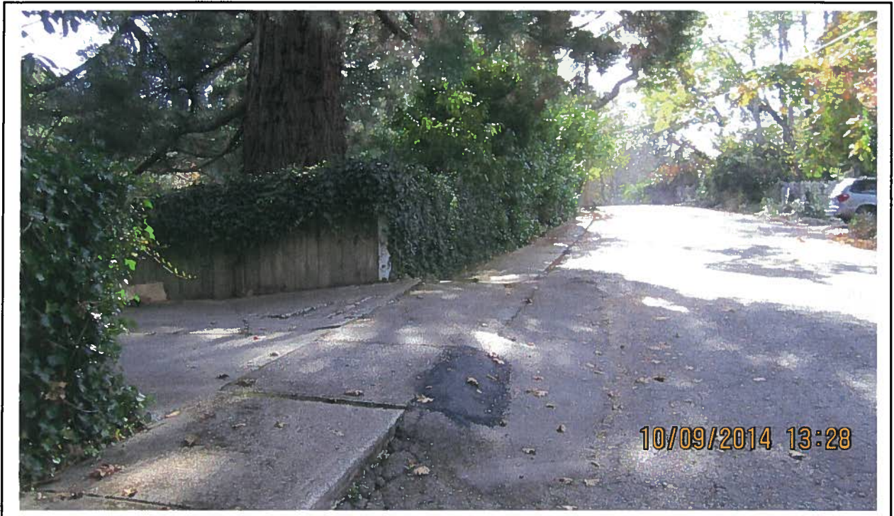
Figure 3: The large private tree causing road damage
